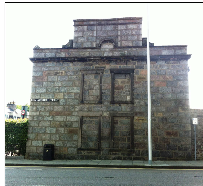
Example of blocked up windows in Ferryhill
